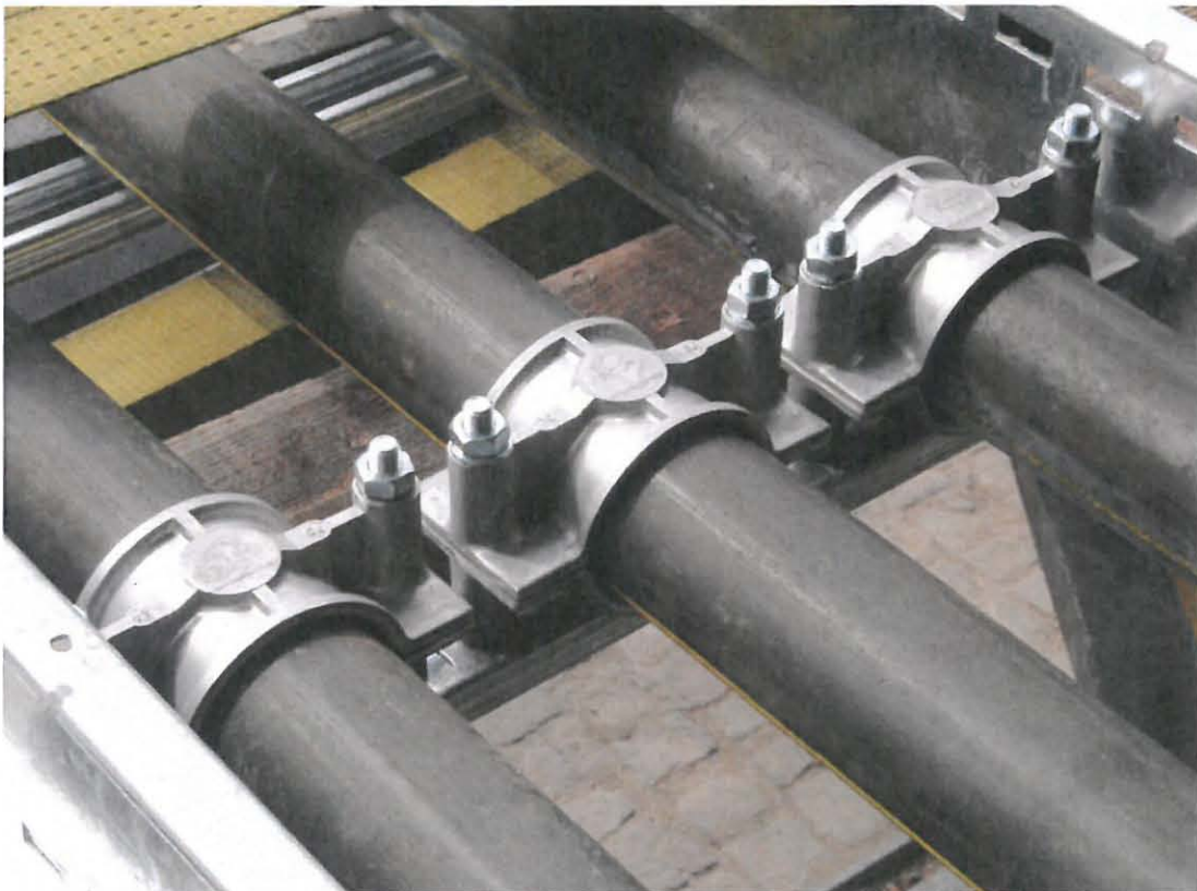
Photo 6 Condition of the tested cleats after the first test
